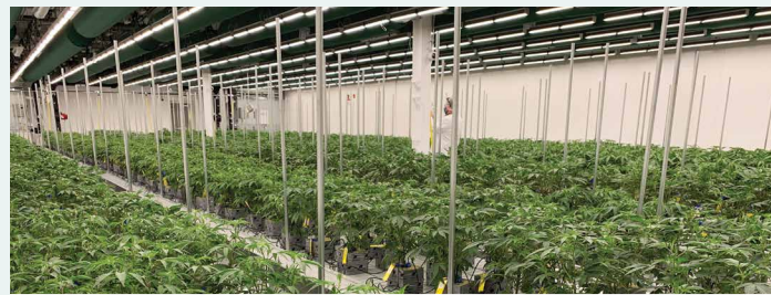
At LivWell, the Argus system facilitates dynamic lighting control so the cultivation team can adjust the intensity of the light over various phases of plant growth as well as simulate sunrise and sunset
