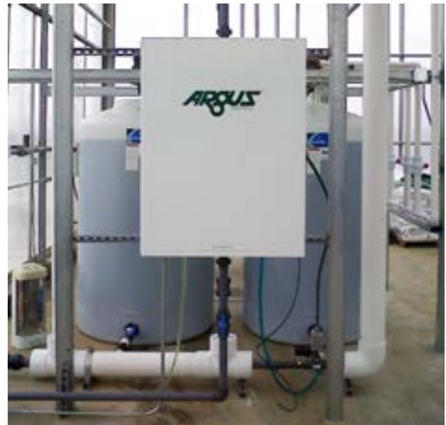
Argus A/B in-line injection system using two stock tanks
